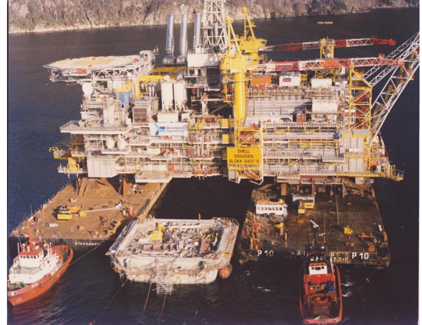
Deck mating by float over – not for the faint hearted. Draugen 1993. 279 m below water, 6 m above! Top side float-over. Sleipner A cracked and sank during trial submergence in 1991
